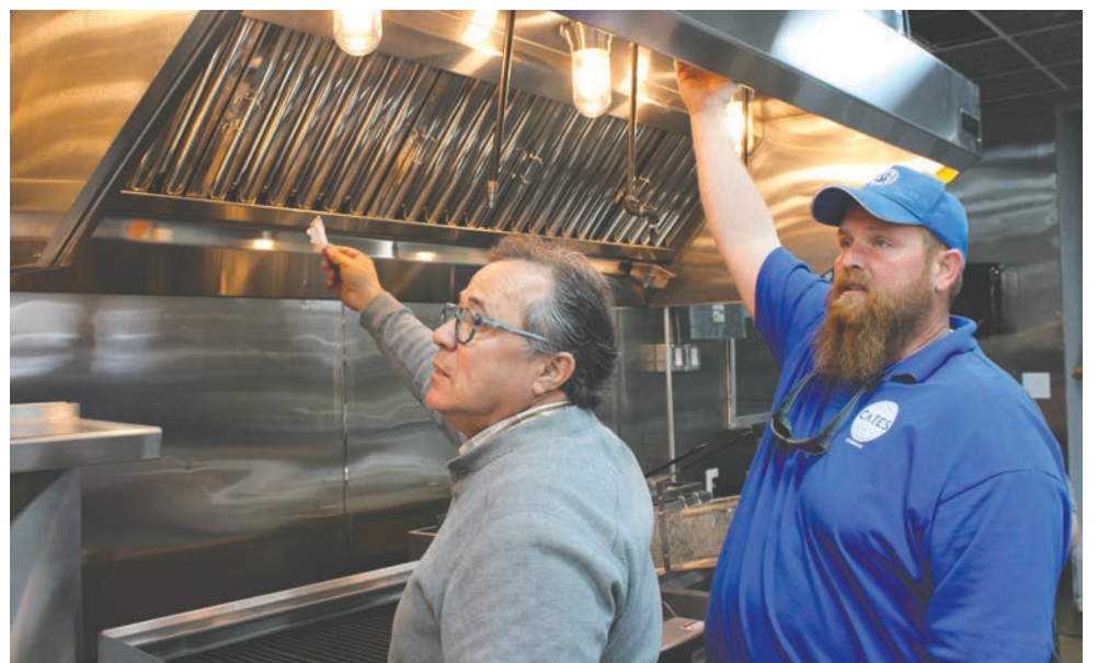
Edward Reese, left, who directs the food and beverage operations for all four restaurants in the Forgotten Coast Hospitality Group, LLC, examines a kitchen fixture with Edward Busby, crew leader for Cates Electric Services, Inc. [ DAVID ADLERSTEIN | THE TIMES ]
