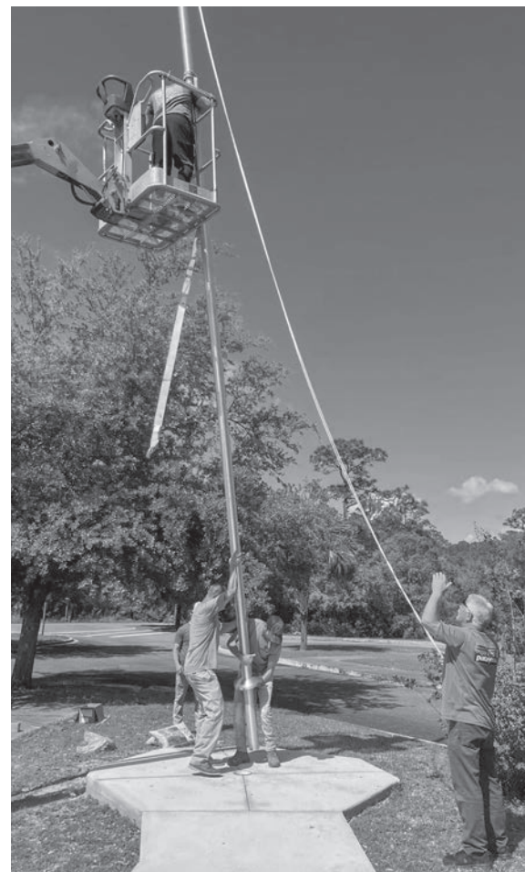
Installing a new flagpole at the Arabella Health and Wellness Center. [JEFF ALLEN | CONTRIBUTED]
