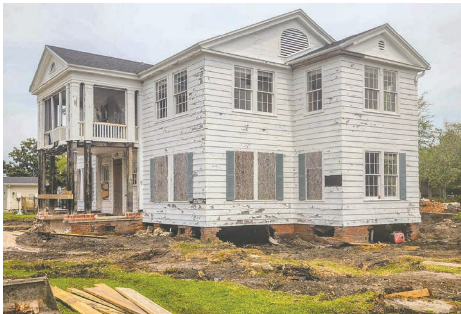
The building has been lifted up and is ready for moving April 17. [THE PORT INN | CONTRIBUTED]
